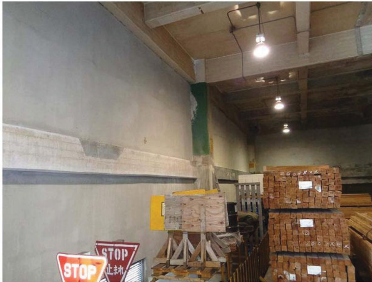
Figure 9 - Section 1 of the ring girder at Building 306 in the Naha Military Port, 2016
