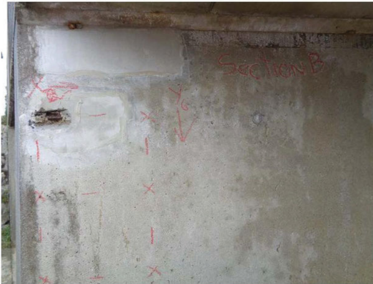
Figure 7 – Sealer still evident after several wettings of the concrete
