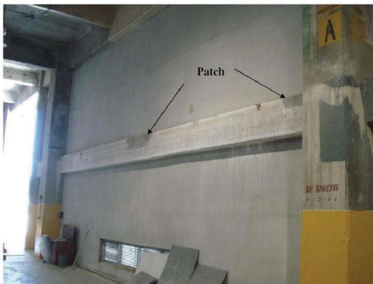
Figure 8 - Section 1 of the ring girder at Building 306 in the Naha Military Port, 2010
